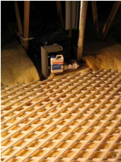
The opened trellis forms an electrical and mechanical safety platform for many types of work and inspection
